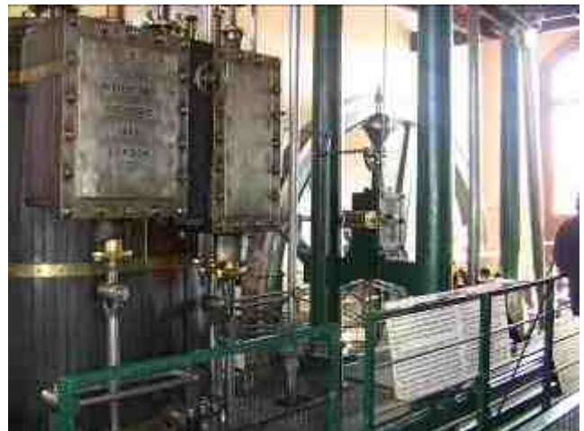
Figure 4 Valve chests for high and low pressure cylinders. Note counter to record number of strokes.
